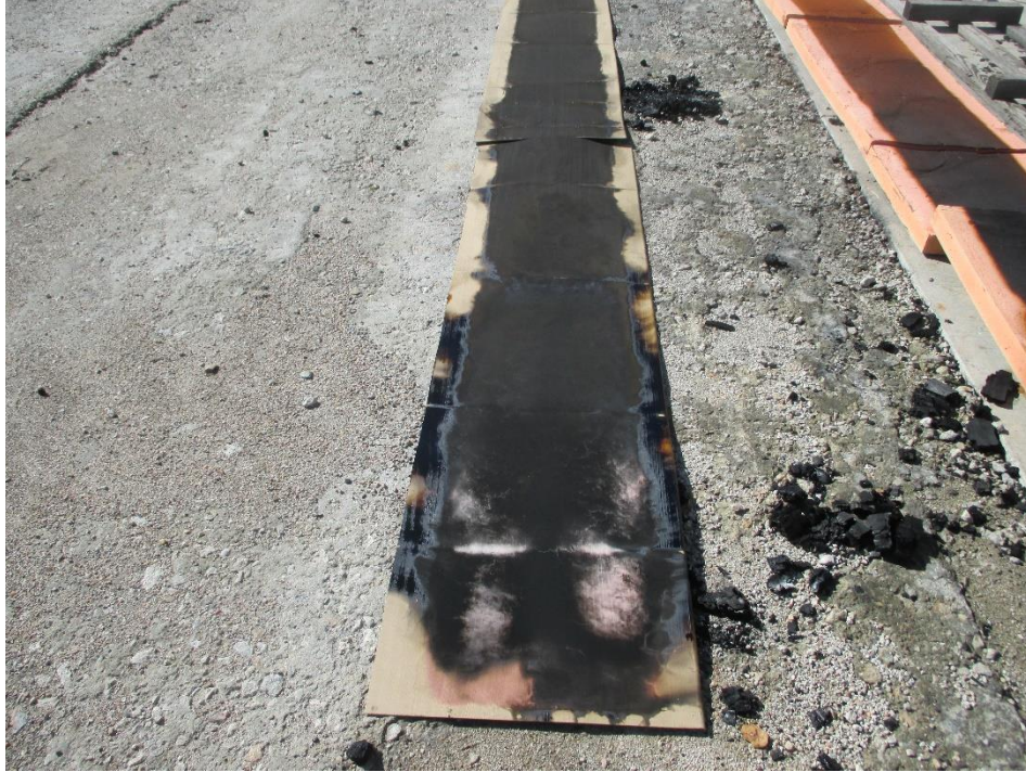
Photo No.5 Post-Test Exposed Side
