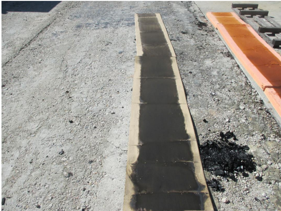
Photo No.6 Post-Test Exposed Side (Continued)
